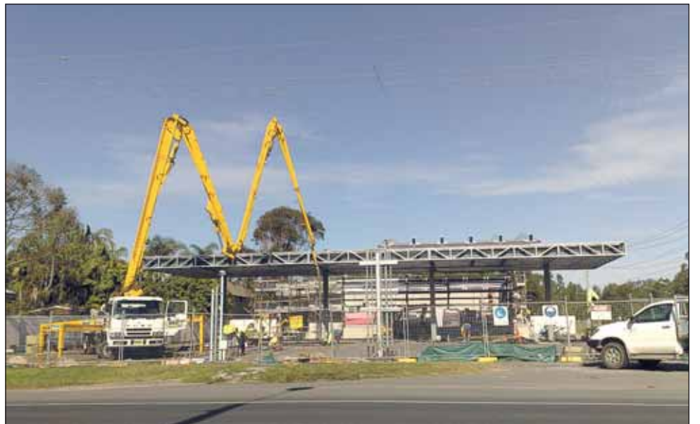
All right, so we were indulging in a little leg-pulling last week with the Whalo-King signs on the former Short Stop site in Byron Bay, but Shane Rennie's picture of the earthmovers seems to indicate that something else might be going on there.
