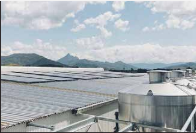
Stone & Wood solar panels provide 10% of power.
