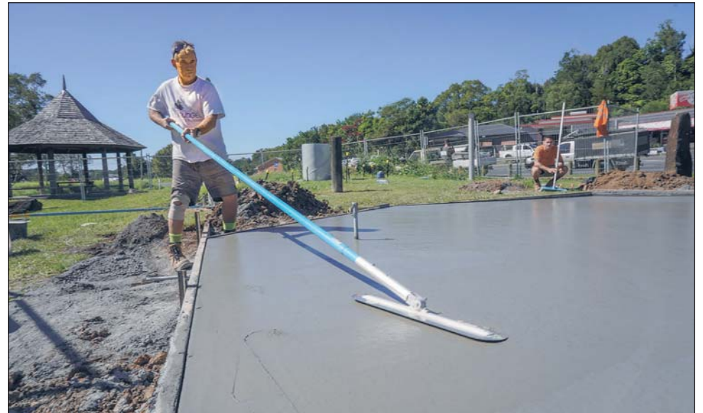
The Mullumbimby Gateway gazebo is being relocated - Daryl Salisbury prepares the slab, which is part of the rejuvenation of the site, which is located opposite Uncle Tom's. Photo Jeff Dawson
