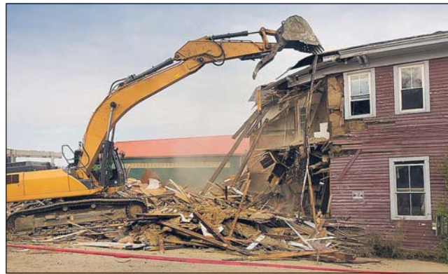
While Council staff have always had powers to demolish homes they consider a risk, the new draft Unauthorised Dwelling Policy 2020 gives greater focus to that pursuit.
