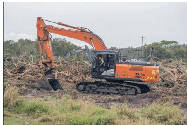
Clearing has begun on Ewingsdale land for the Harvest Estate project, which is owned by Tower Holdings.
