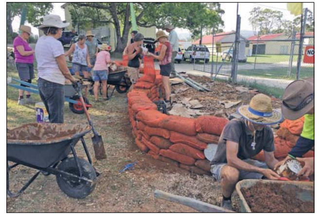
Community earth building day, Murwillumbah. Earthbag technique is used here, a robust and simple earth construction technique. Photo Rebecca Whan
