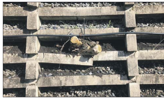
Damaged wall at Bangalow. Photo Roger Seccombe
