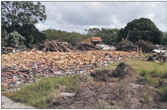
Fourteen perfectly-liveable units on the site donated by Florence Price to Ballina Council have been sold then demolished. Photo Alan Nicholls
