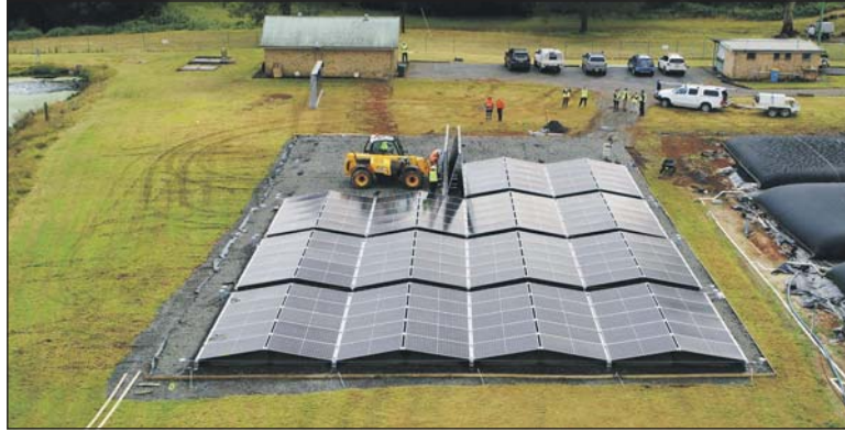
Ballina Council's Alstonville WWTP solar panels.
