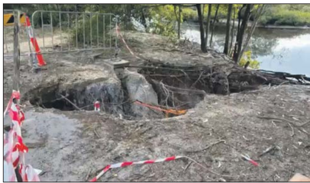
Some of the remediation works urgently needed along the Brunswick Heads foreshore. Photo supplied
