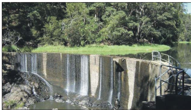
Lavertys Gap Weir which supplies water to the Mullumbimby Water Treatment Plant. Photo NSW Govt OEH
