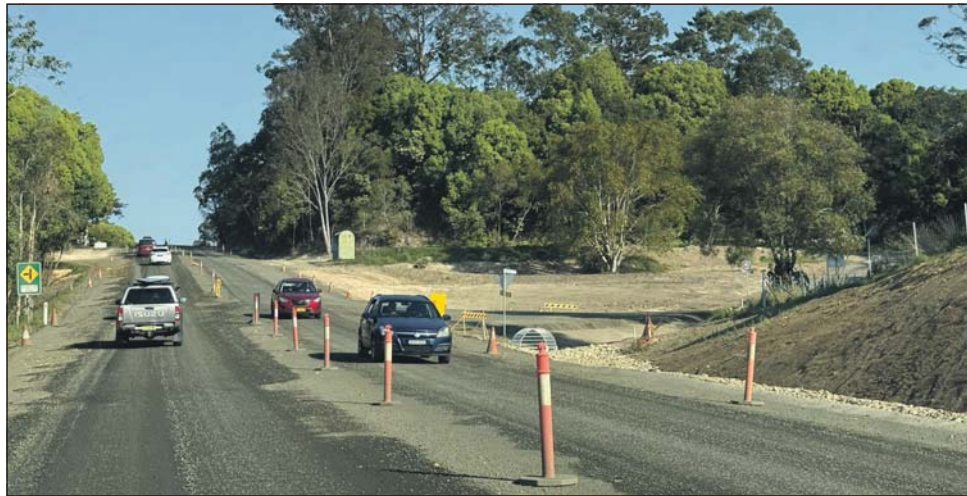
The Maculeys Lane and Mullumbimby Road intersection. Get ready for a massive disruption to Mullumbimby's outbound traffic to the highway over the summer break. Photo supplied
