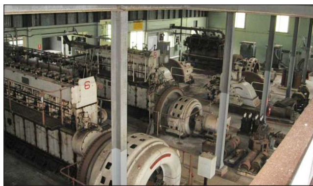
View of power station floor showing later diesel generators with original hydro turbines to rear. Photo wikipedia.org
