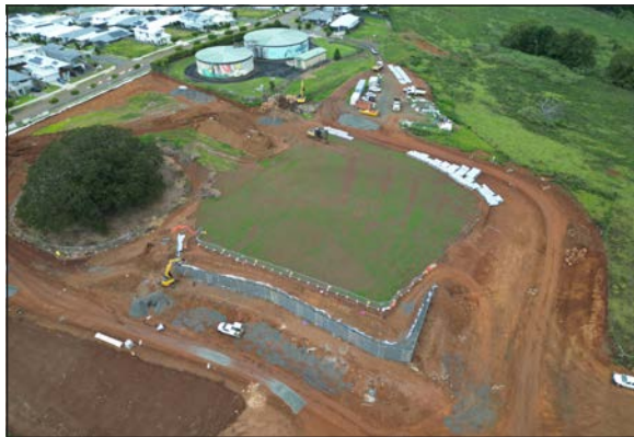
Construction of Banyan Hill's landmark Hilltop Park is progressing, with completion targeted for mid-year.
