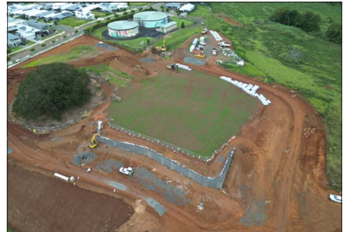
Above: Construction of Banyan Hill's landmark Hilltop Park is progressing, with completion targeted for mid year.
