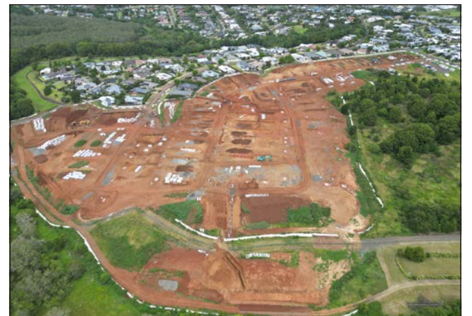
Above: Construction of Stage 10 and 11 is progressing well and on track to practical completion in July 2026.
