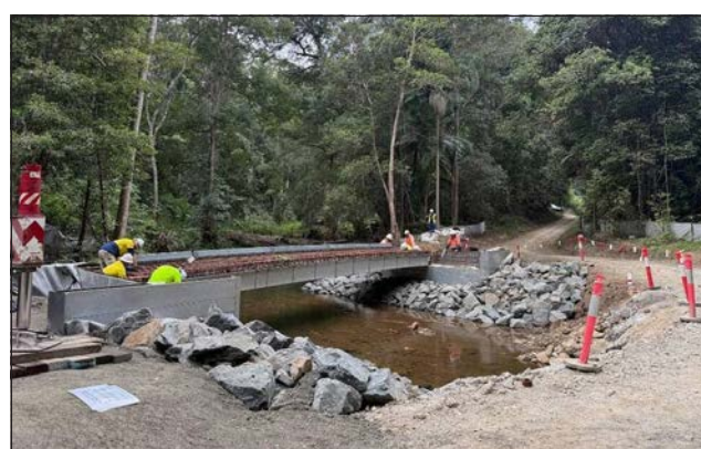
Bridge construction at Rowlands Creek, between Main Arm and Uki. Photo Tweed Council
