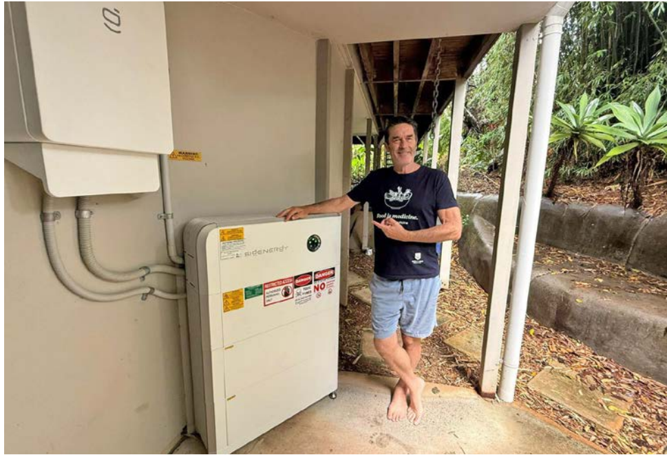
A rooftop solar system combined with battery storage provide this home with clean energy. Photo Mandy Nolan
